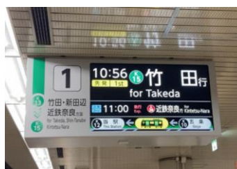
Renewal and installation of train information display equipment on the Karasuma Subway Line
